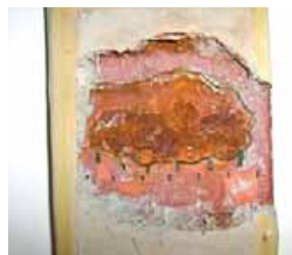
Another commercially available epoxy passive fire protection product showing extensive corrosion creep (>10mm)
